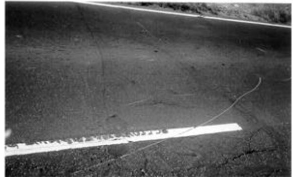
Figure 5. Semicircular scratches on the pavement produced by the lance cross the central line of the route.
