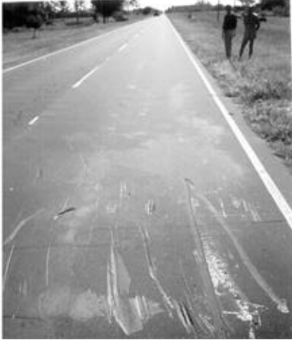
Figure 3. Overview of the two lane road at the crash site The marks in the pavement indicate the place where bus and trailer impacted.
